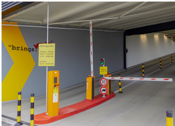
Barriers at the entrance and exit control the traffic flow on the site.
