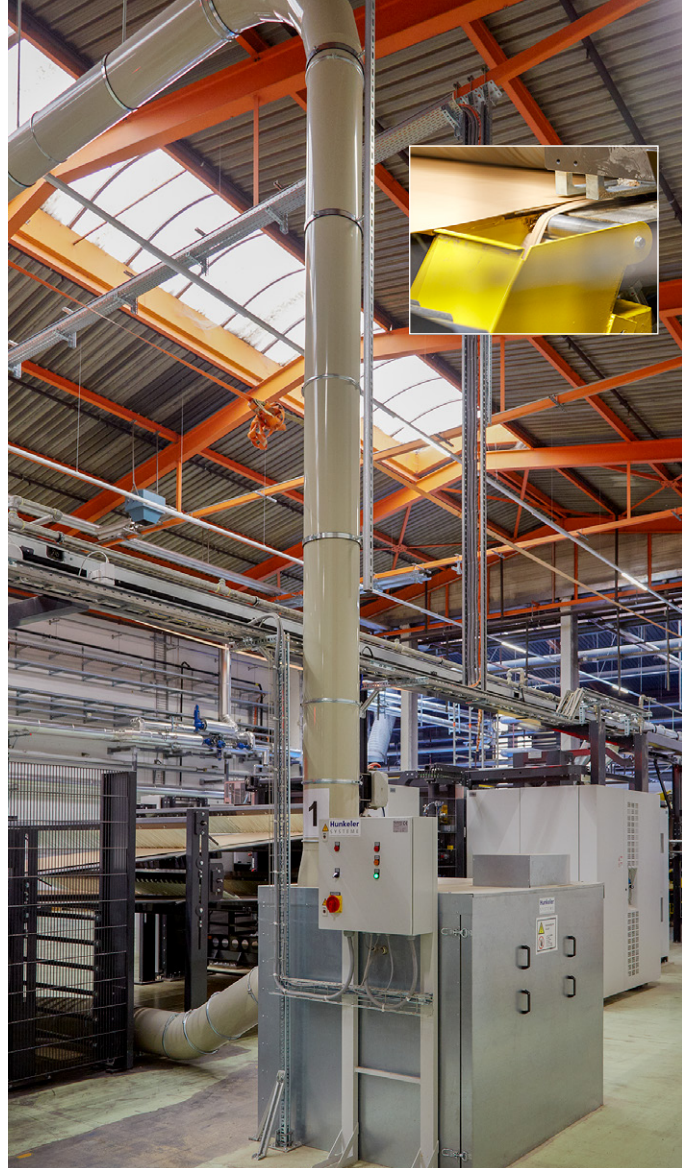
The edge trim extraction system (small image) and a chopper fan ensure the operation of the corrugated board plant.
