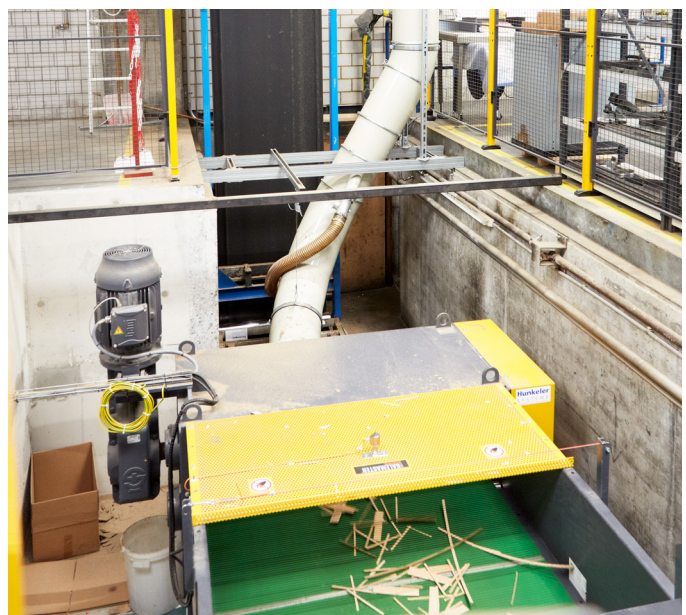
For the disposal of cardboard waste from several converting machines, a high-performance shredder, fed via a conveyor belt, is integrated into the system.
