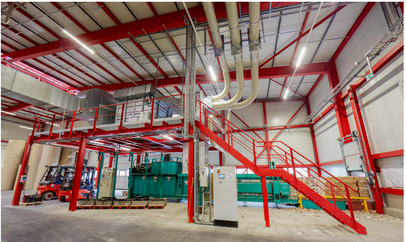
The entire extraction system is space-efficiently arranged on a second level above the baling press.
