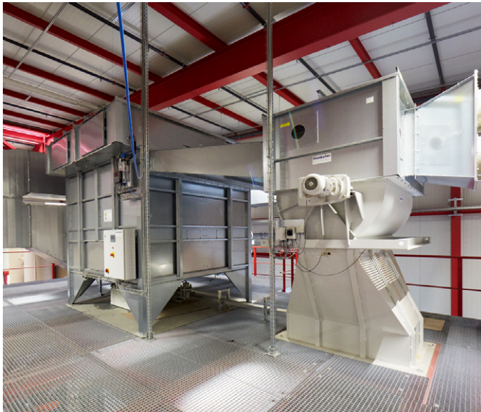
A compact extraction system consisting of a separator, a filter, and a fan with an energy-saving system ESS forms the heart of the installation.
