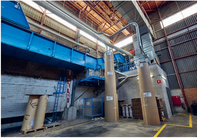
A large-scale disposal system ensures a continuous process in corrugated cardboard production in 24/7 operation.
