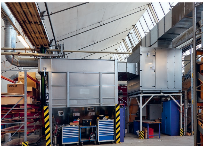
The edge trim, intermediate trim and die cut grids that accumulate during the processing operation are removed from the production area via extraction technology and conveyor belts and fed to the baling press.
