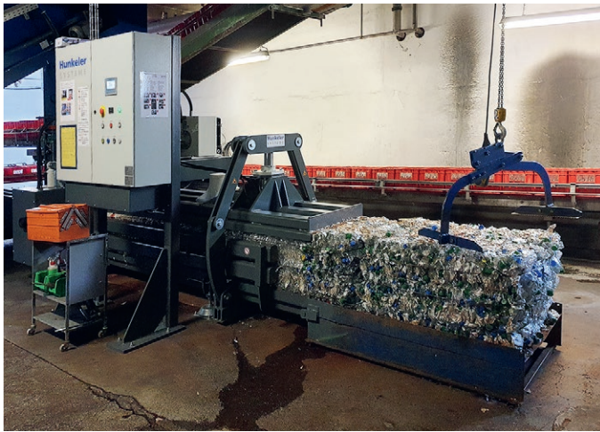
A new PET baler with a Compactor module replaces a system from 2005.
