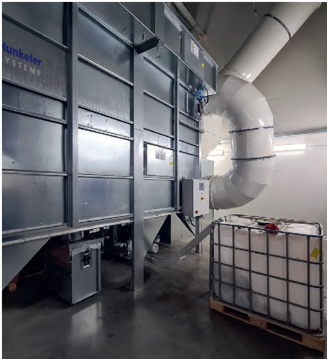
The technology operates according to the proven negative pressure principle, with the fan located at the very end of the line.
