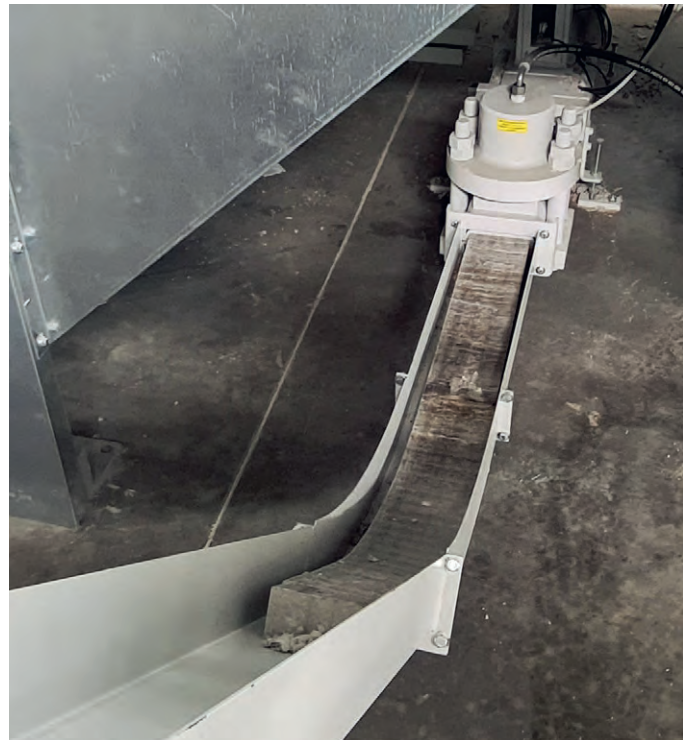
The paper dust leaves the extraction and filtration system in the form of compact briquettes.
