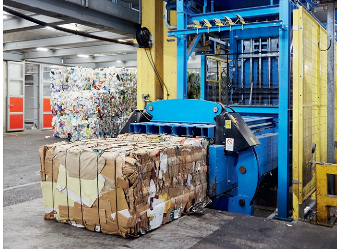
In Dierikon, over 6000 tonnes of material (cardboard, PET, PE and plastic films) are compacted into bales every year on the press.
